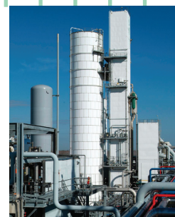
Large air separation unit and pipeline system
