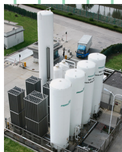
On-site gas generation
